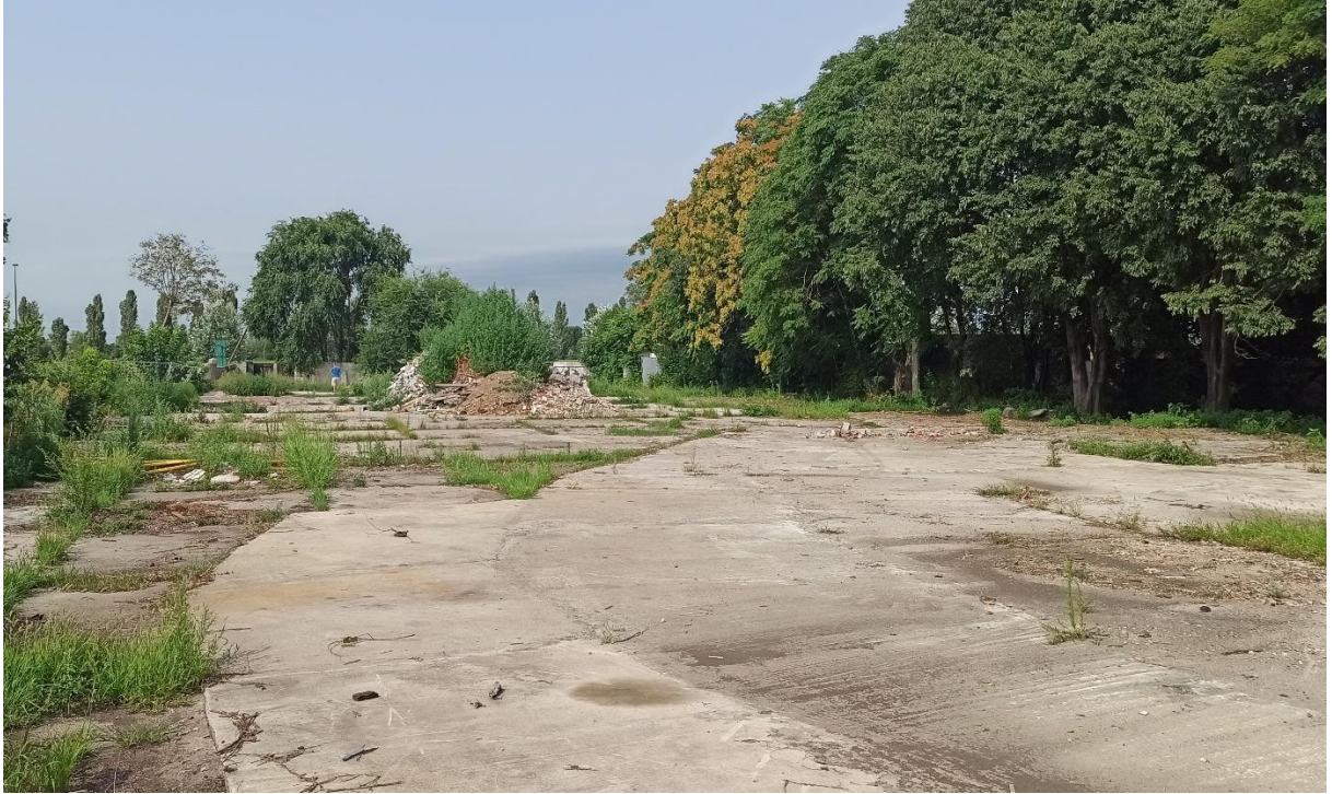
Figure S1. Experimental site with concrete pavement prior to desealing operations (September 2023).
